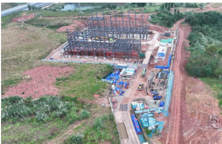
图3-3变电站区无人机航拍
