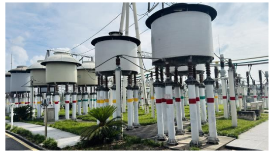
35kV 低压电抗
