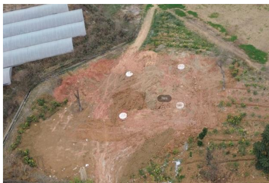
NA24塔位扰动裸露表土未覆盖
