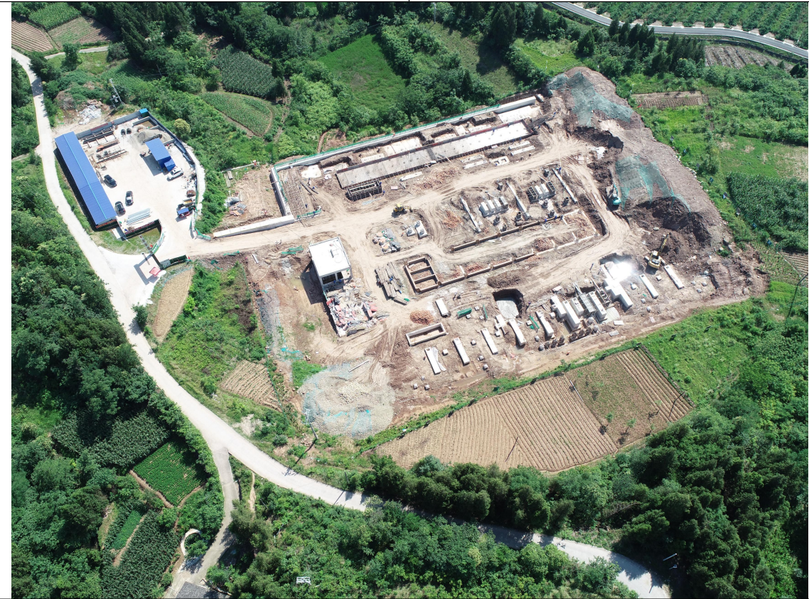
阆北变电站-无人机-现状
